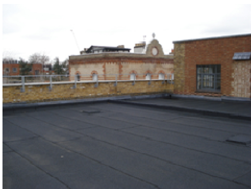
GENERAL VIEW OF ROOF/ SECOND FLOOR LEVEL TO 22-26 STANNARY STREET LOOKING NORTH WEST
